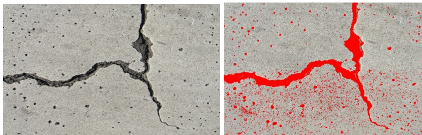
(A) Original data (B) Segmented crack by red color
